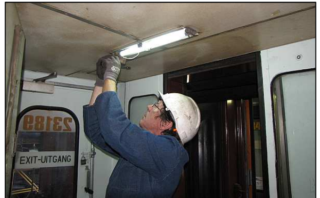
P166 - Reefsteamers' coaches have all been converted from the complicated DC axle generator-and-battery setup, requiring inverters, to using a standardized 3-Phase system using modern 220V fittings. This also means that our coaches can be easily powered by standard electrical power at trackside and by generators.
