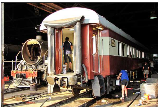
P167 - Because of the sheer size of a railway coach, projects such as floor repairs and painting require the efforts of a full team to make any progress.
