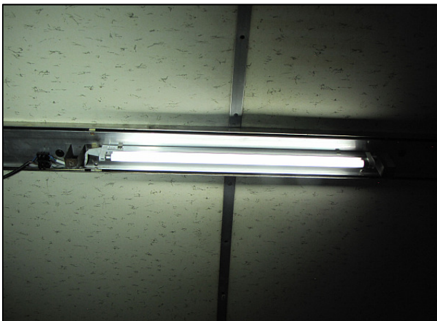
P05 - The lights in the main cabin have already been upgraded to 220V high-efficiency tubes with integrated electronics. The water pumps will need to be replaced.
