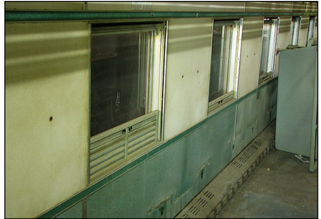
P04 - The louvered shutters are going to be removed and relocated to our sleeper coaches, where they are of more use. The louvered corner skirting and the steam heating pipes within will be removed and scrapped to allow for a clean edge to the flooring.
