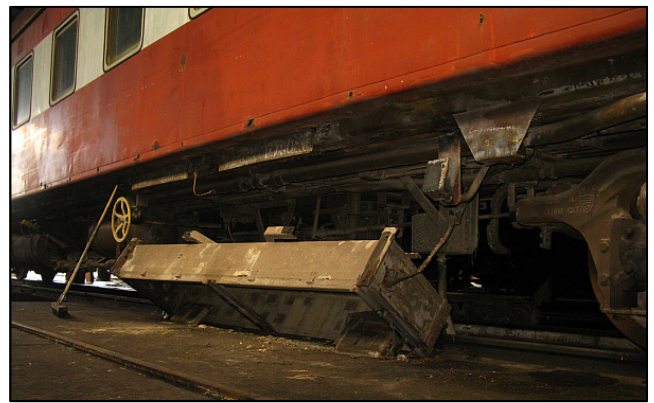
P10 - Underbody clearing is getting under way between other jobs. This is an old fibre-glass battery box that has just been cut away. Obsolete equipment is cut away to reduce weight and clutter, and to free up space for the fitting of new equipment – including the planned sewerage cess tanks. (And extended water tanks for the sleepers.)
