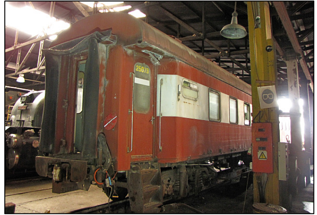
P02 - Some of the hardest work to be done is the repair of the exterior sheeting which is perforated due to the corrosion of coastal air, and the years of using steam heat. Stripping has already commenced on the obsolete steam heating and electrical equipment 'under the decks.'
