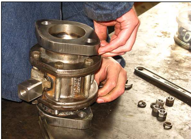
P19 - As the flanges are very close to the valve body, the clamping bolts all needed to be cut down and their threads manicured. This photo shows the new square-shanked noggin and the existing valve stop plate. The old SAR valves could rotate through 360 degrees but would only seal properly in one orientation. To add to the confusion, the original kick lever shafts can be pulled upwards to disengage them and refitted in any one of four orientations.
