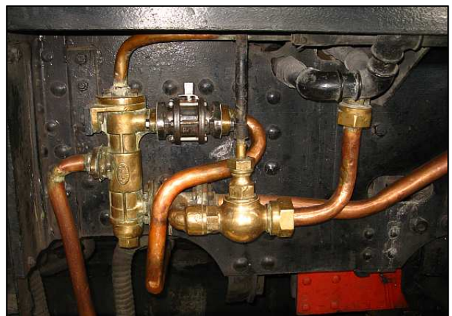
P30 - The tweaked pipework fitted to the new valve. The steel valve doesn't look pretty amongst the antique copper and bronze - but utility and reliability overrides aesthetic considerations. Best of it is that we can easily revert to the old valves if this doesn't work out as planned.
