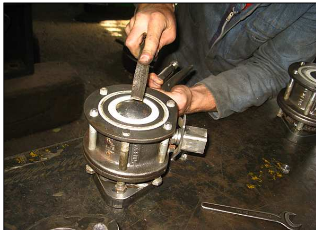
P20 - The bolts were being incrementally ground-down with a mini grinder rather than being sawed off. If you look closely at the photo, the pairs of bolts to the left and right had already been chamfered and cleaned. The remaining two bolts had to be cut down quite precisely as their axis conflicted with that on the main flange bolts. (Unavoidable because of the valve/flange orientation.) Enough thread had to be left to allow the nuts to tighten up properly.
