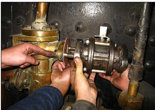
P23 - Test fitting the valve. They knew the adapted flange would match, but the bolt being pressed inwards was still unknown. It turned out too long and had to be trimmed even more. Which pair of hands belong to which grunt?
