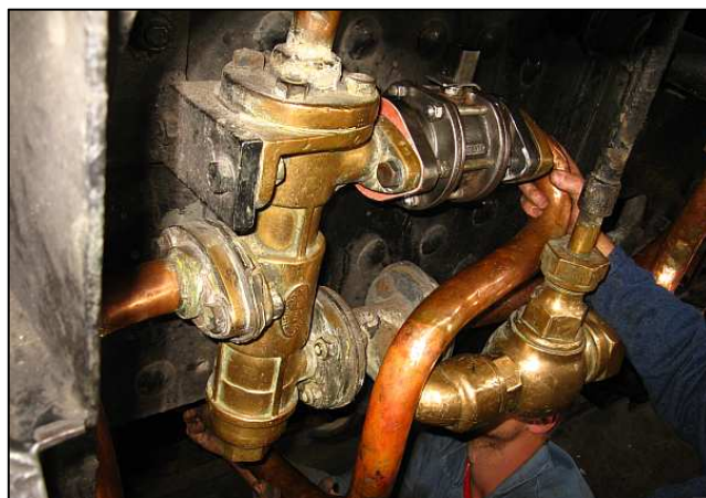
P24 - Now THIS stage of the job was the most awkward and swearword-inducing. Not only did the pipe flange need to fit, but also the intake elbow at the bottom, with the pipe making a longer swan neck around the drench valve.
