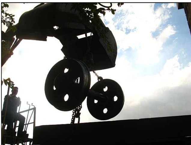
P17 - The final lift went with ease as the weight of the axle was well within the boom's capability for the radius at which it was reaching.
