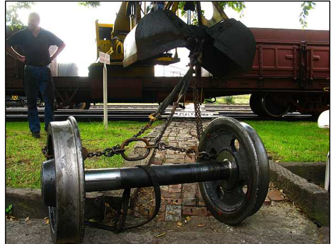
P14 - I took a quick snap of this contraption and then got smartly out of the way as the tension built up – the axle would have to be dragged first. We often use a wire cable sling wrapped around the clam shell grab's impulse bar as a base for shackled chains and slings for hoisting.
