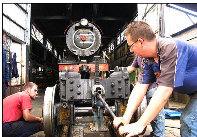
P12 - Almost at the limit of the jack and trying to get enough space for a sleeper to cross the track under the frames. Jeandre is watching the bearings as when the brasses are released, they can just pivot freely around the axle and fall off, like a horse shoe being rotated on a broom stick.
