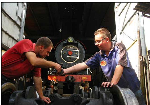
P05 - Team work ... gimmie that nut and washer before they get kicked amongst the fallen autumn leaves and lost!
