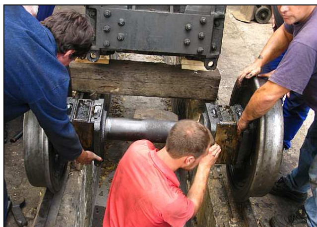
P16 - The front axle is now completely out and being rolled carefully towards the viewer. Notice how Dawie (L) and Jeandre (C) are supporting the bearings against the counter-drag of the rotation. Dawie needed a more secure grip as he had the damaged bearing with the grooved axle journal applying more force.
