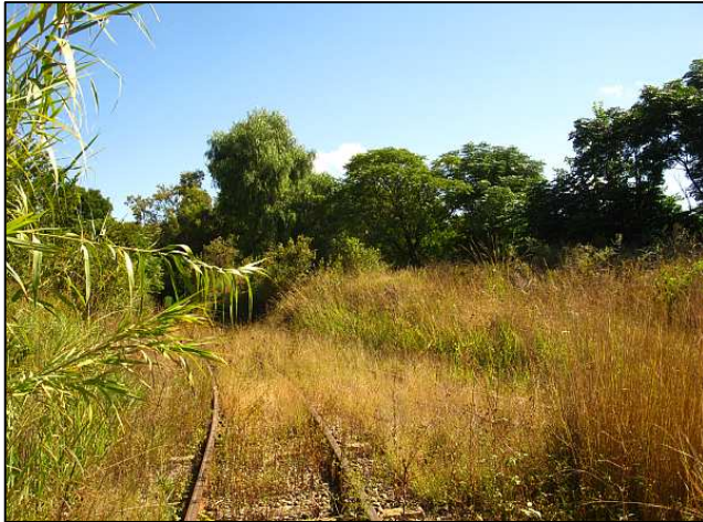
P01 - After a long warm, wet summer, the Magaliesburg turning triangle had become overgrown and the points all gritted and rusty. While Transnet will look after the major repairs such as alignments and sleepers, Reefsteamers volunteers will now need to keep the foliage under control.
