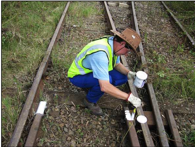
P09 - Alan Lawton paints the tips of the guard rails on the points, as per the standards required to be kept within the Germiston Depot Yard.
