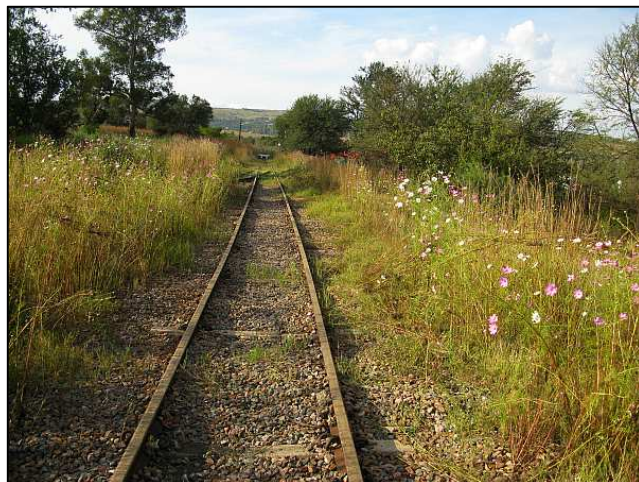
P18 - The 'final product.' A nicely cleaned length of track plucked by Jannie Gouws and little me, and then skinned with Bongani and the Weedeater. Reefsteamers needs to take over the triangle from now on, so we need to plan for a spring weed spraying and an mid-autumn burn-off.
