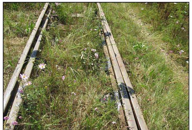
P06 - All of the points had their pads cleaned and liberally lubricated with heavy graphite grease. It was applied with a brush, so grease on the railhead was inevitable. The rail heads will need to be cleaned before the next usage.
