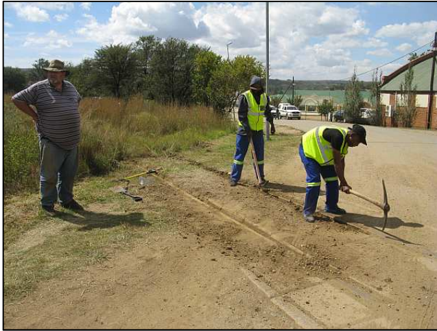
P07 - Work starts on chipping out the grooves in the level crossing. Although the fill was 'only' soil, it had been baked quite hard and repeatedly compacted by the road traffic.
