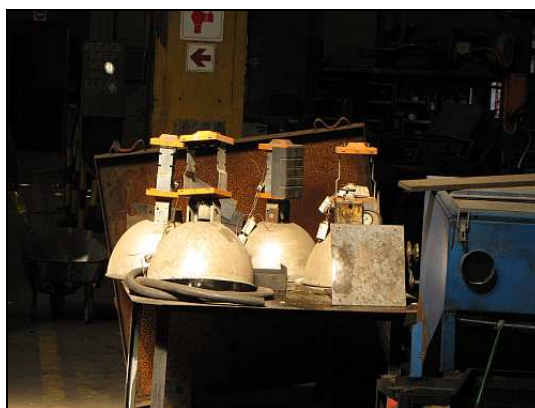
Some of the old lamp fittings awaiting conversion. Essentially, the old ballasts and extra wires need to be removed as the new 'twirly' CFL lamps operate directly from the mains.
