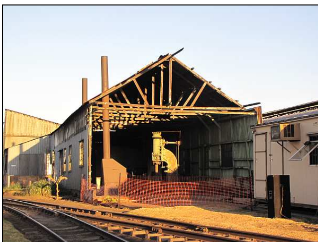
P27 – The old steam hammer and the outer forge in the stripped-out forge shops catch the rising sun as well. That orange safety netting, although ugly, was quite effective in keeping people out of dangerous areas. It is much better than stripy tape and we will definitely use the idea again.
