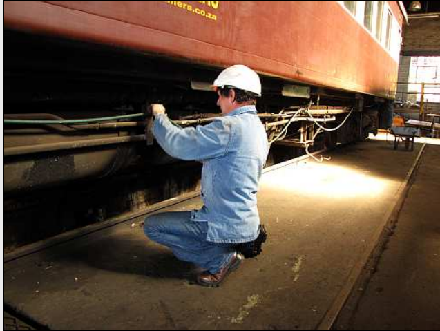
U01 – Alan snips away a cheap green nylon garden hose that ran the full length of the coach. It was used to transfer water along a coupled train and serves no purpose since the pumps are all functional.
