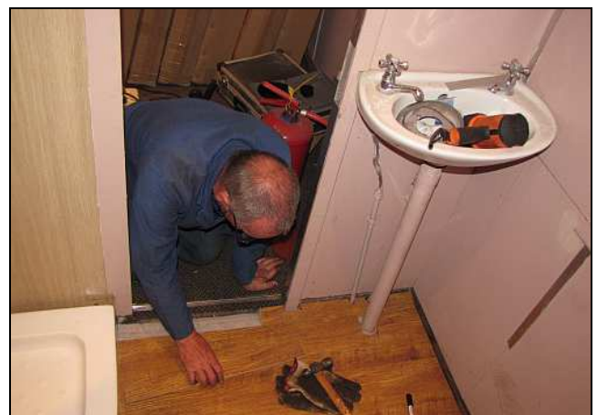
S06 – Gordon fitted the notched plank that custom-fits around the pipes even though we will have a pedestal under the sink. The little gaps around the pipes, especially the drain, will be filled with puddled silicone to floor height.
