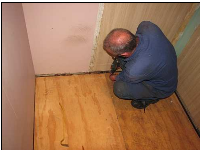
S11 – Gordon zaps in yet another self-drilling screw – these were even able to go through the fireproofing steel sheet in the middle of the bulkhead walls. The floor bowed upwards a bit in the middle and is now under compression.
