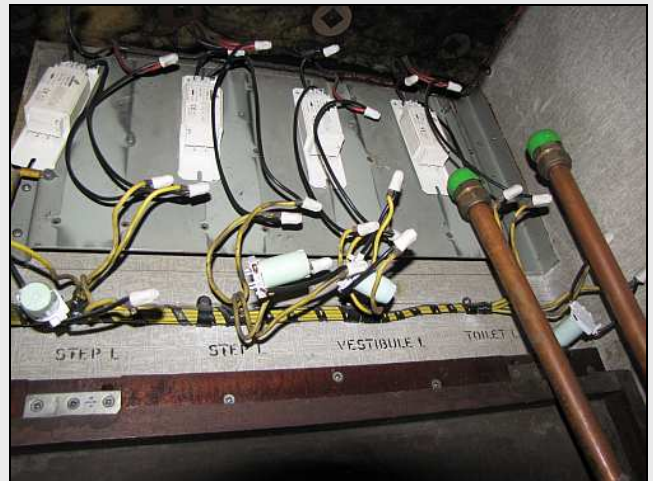
X04 - Looking into one of the wiring chambers above the geyser cupboard. The copper pipes are capped with vacuum breakers, which is good, but they are in direct contact with the live wiring, which is bad news. Shaun Ackerman was happily investigating and poking around with his hand in the semi-darkness, but he withdrew rather quickly as soon as Alan shone a torch in there!
