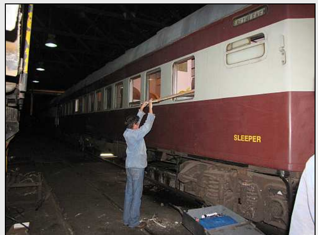
S18 – The plywood boards were sourced from a dismantled model train layout, so it is kinda appropriate that they find a new home on a REAL train! Any items going onto a Cape Gauge passenger coach has to fit through narrow corridors and doorways, or through the windows. Mr. Maurer has already taken note of this restriction for the new furniture!
