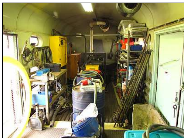
P44 – The optimized and ventilated generator room was a great success. Even with the large John Deere engine running, it was actually cooler in here than in the coach compartments. The generator ran without problems.
